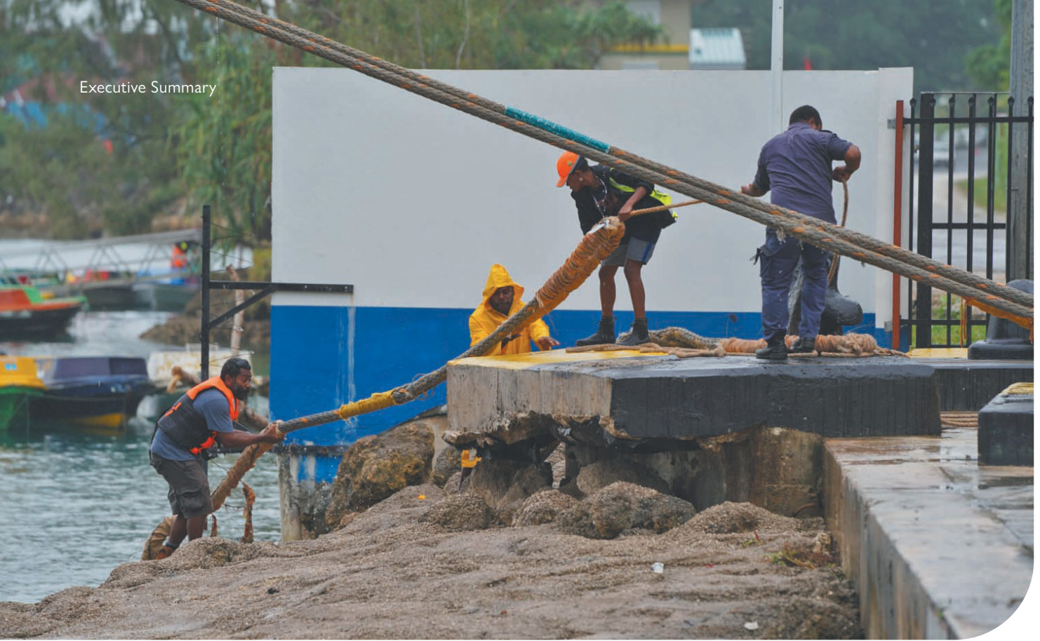
Ni-Vanuatu workers fixing up the sea port area in Port Vila. © IOM 2023
